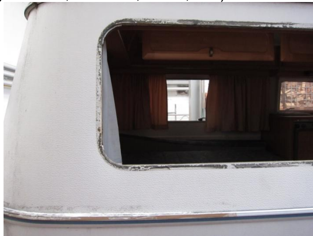
An overview of three possible weak points: roof sealing, window sealing and assembly weld upper to lower trailer body The reason here: old and porous window sealing
